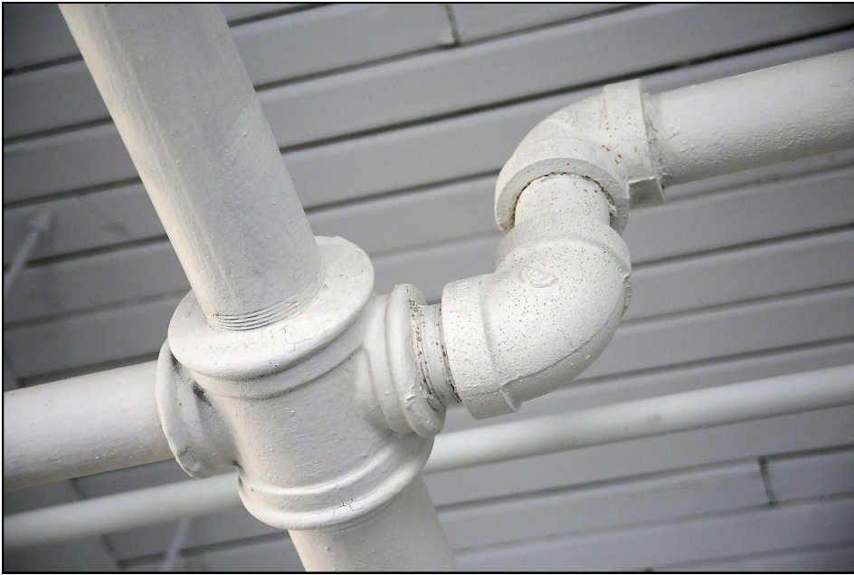
Figure 6. Water and sewer pipes can run against basement walls or come down somewhere in the middle of the basement.
